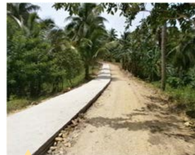
A Road of Opportunities. Through the Grassroots Participatory Budgeting process, a dream is realized—photo shows a farm-to-market road being constructed in the town of Mulanay, Quezon to help facilitate mobility of people and farm produce. (Photo from RIU)
