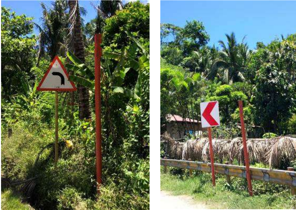
Figure 22. Poles with missing traffic signages
