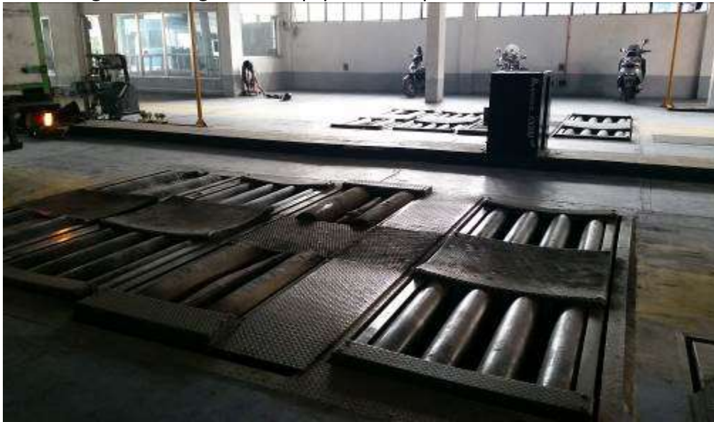
Figure 10. Stage 2 Test Equipment Peripherals: NCR North MVIC
